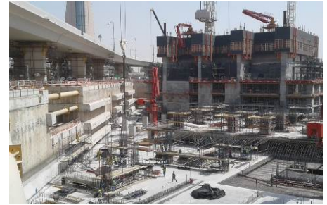
Geotechnical and Geodetic data from a deep excavation, existing bridge and high rise building
