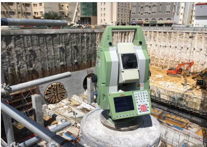
Real time geodetic monitoring from an underground station of metro
