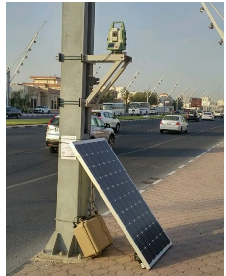
Geotechnical, Geodetic near real time data monitoring, in correlation with TBM data, for Gold Line, Doha Metro, Qatar
