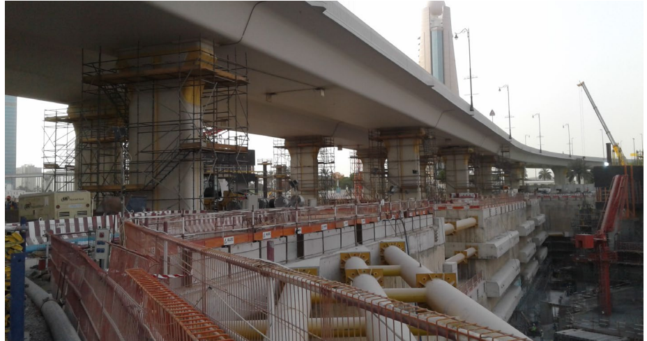
Online monitoring of existing bridge, deep excavation and new structure construction, with geotechnical and geodetic instruments
