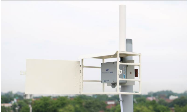
Figure 2-5 EWN-01V VV node mounted on mast with a protection box (antennae inside protective tube)
